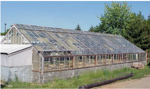
Before: greenhouse in need of repair
